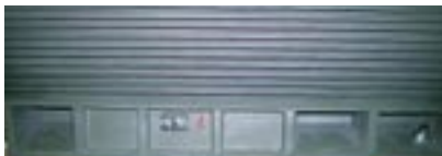
Grounded cast iron stator
