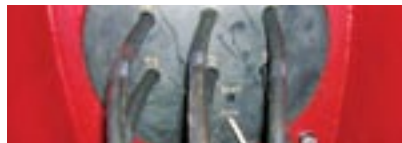
Clearly labeled, separated, and gasketed leads
